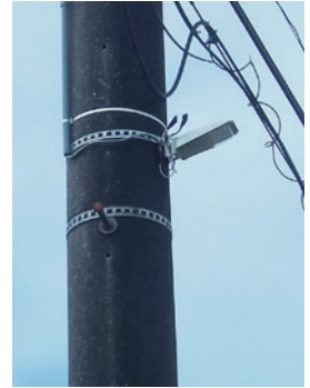
村内設置の防犯灯
